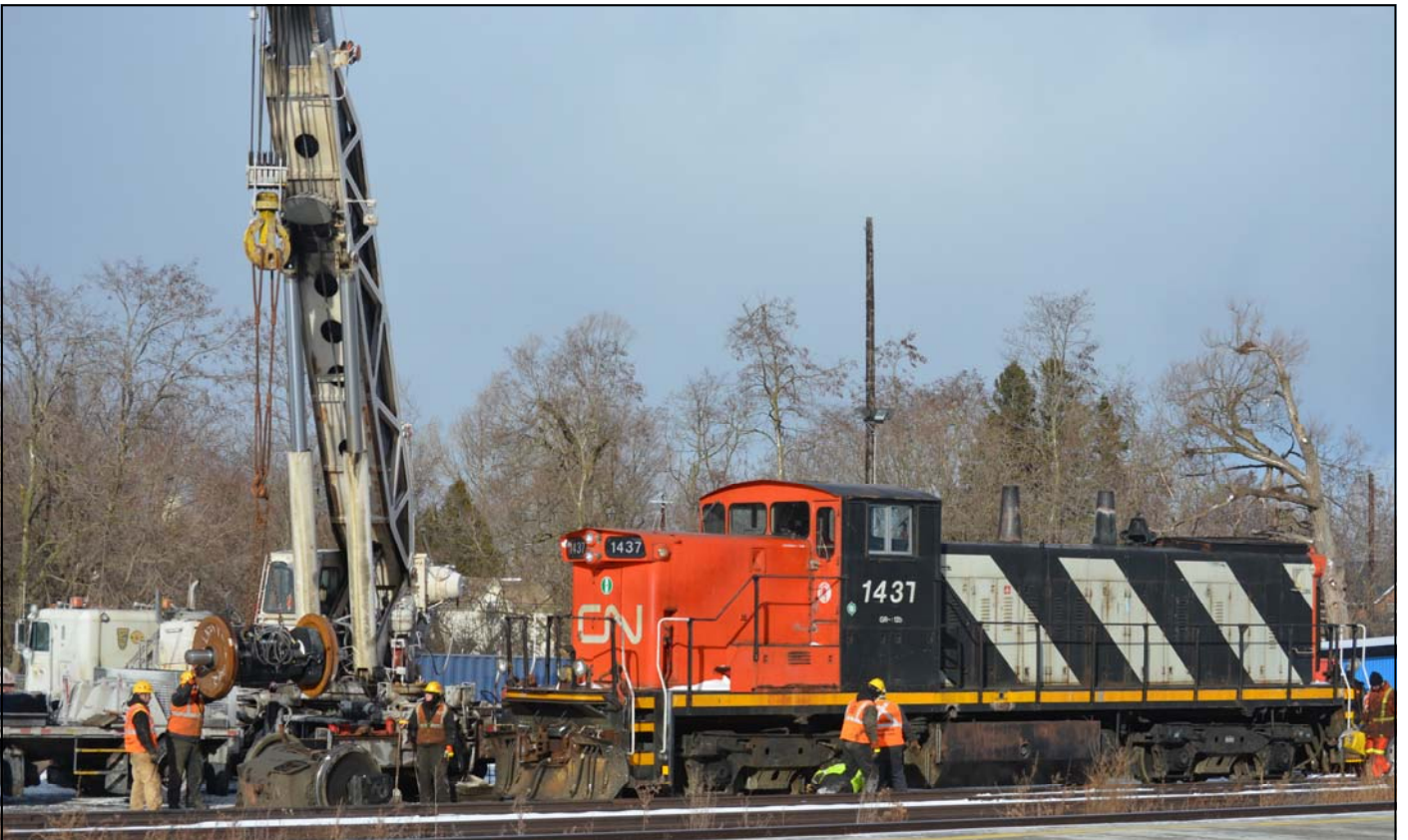
PHOTO BELOW: The damaged traction wheel set on the ground, the new one is being swung over to be set on the track in front of 1437. The cab end will then be raised again and the traction wheel set moved underneath the cab.
