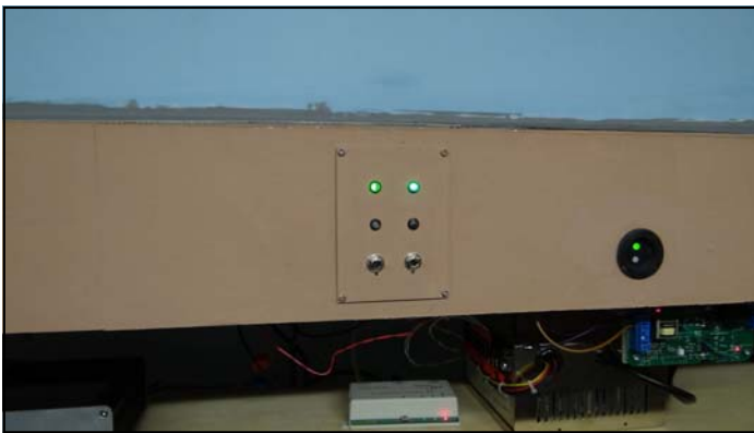
PHOTO 4: Power district controls: Controls for two adjacent districts are shown. The left is for the Rexdale area industrial tracks and the right is for Etobicoke North. In the event of a short circuit in either of the two districts, the corresponding lower LED flashes red and an alarm sounds. The alarm is turned off and power restored to the sector with the toggle switch. The PSX circuit breaker for Etobicoke North can be seen below the fascia to the right (below the Touch Toggle)
