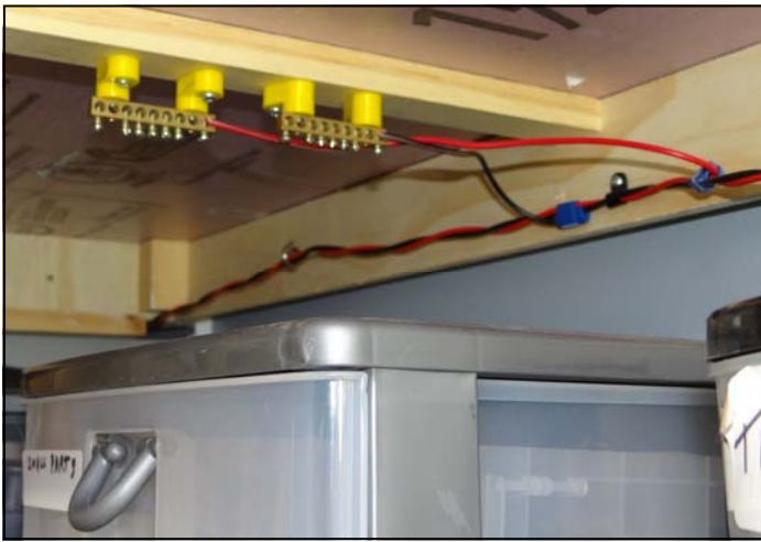
PHOTO 3: The DCC (Lenz) 14 AWG bus: Track feeders (22AWG) will be fixed to the brass connectors about every 120 cm. of flex track.
