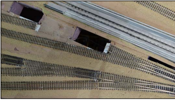
PHOTO 10: Installing the turnout assembly: Holes cut for installation in the MacMillan yard. The tracks in the yards and the industrial spurs are laid directly on the Styrofoam base (the track in the upper right without ties is for an engine inspection facility).
