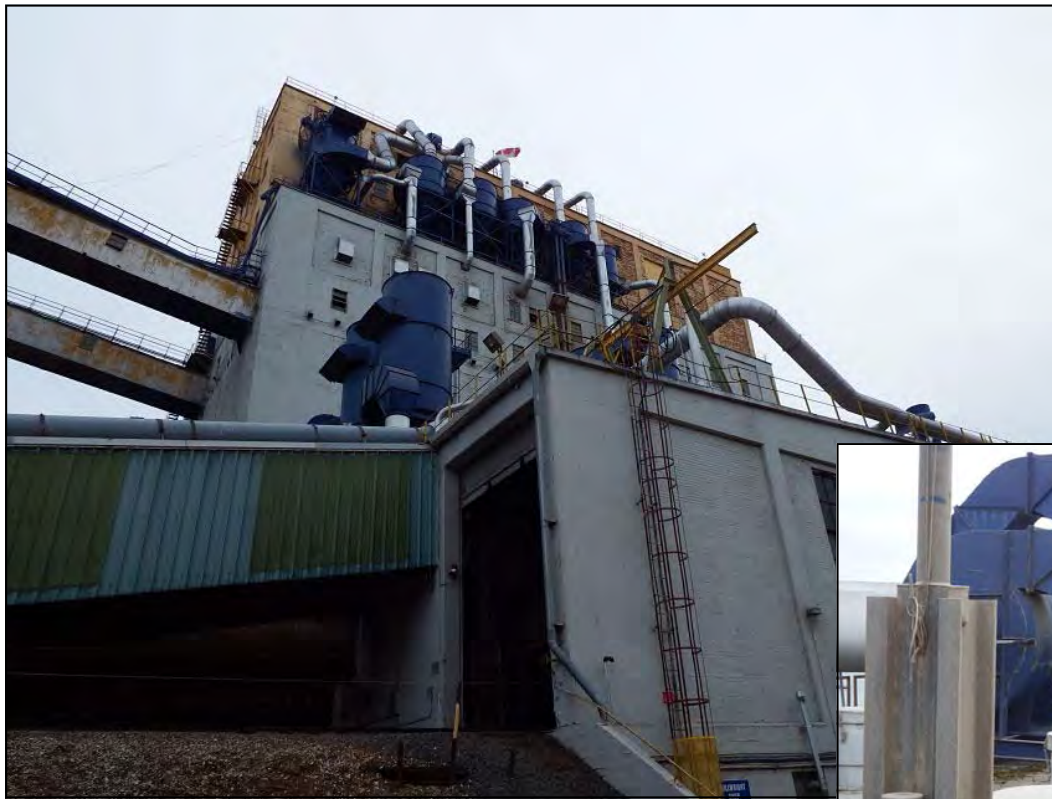
Photo Left: Walter Reid photo: Exterior view of the Richardson Terminals Elevator clearly showing the dust collectors.
