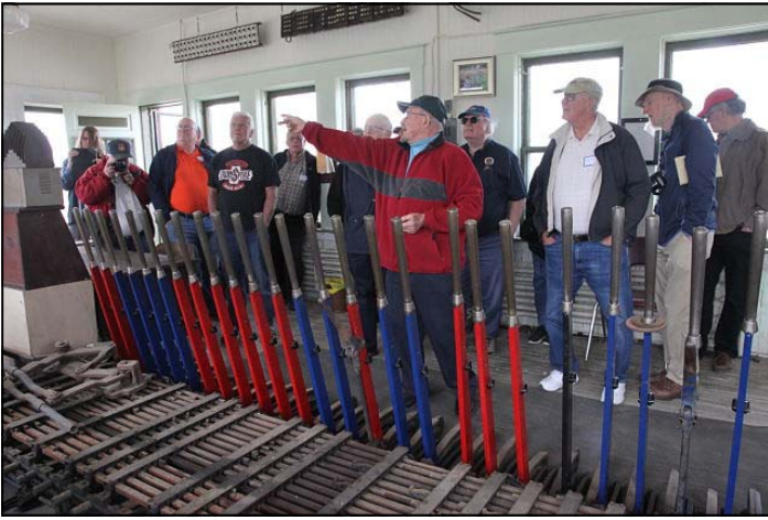
PHOTO ABOVE LEFT by Gerald Harper: Elgin County Railway Museum BX Tower former operator Charles Beckett demonstrates the interlocking switch and signal levers.
