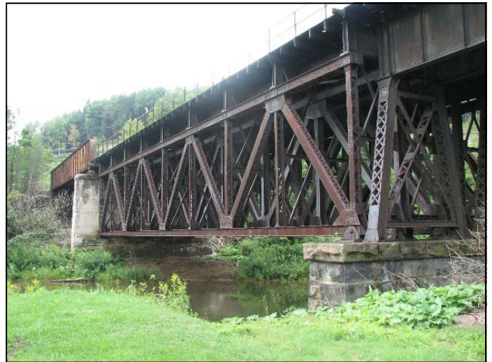
Photo above: Looking south at the railroad trestle as it crosses the Clarion River.
