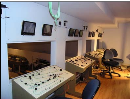
Photo Left: By mid-August, 2013, the control panels were installed. Each panel (there will be six altogether) has TV monitors connected to cameras in the ceiling, so all uncoupling magnets are easy to spot. After all, the distant part of the layout is eighty feet from the operator.
