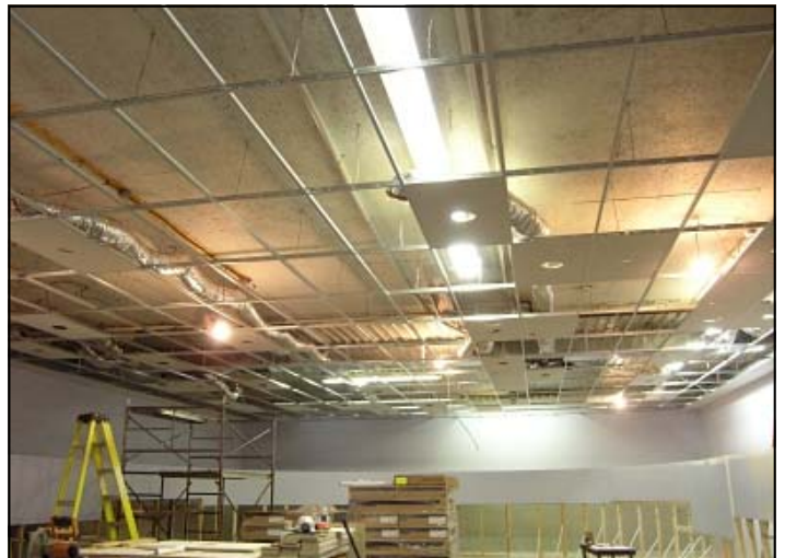
Photo Below: After stripping the building, we constructed a room to match the old one, installing HVAC ducts, cameras, and lighting as the ceiling was installed.
