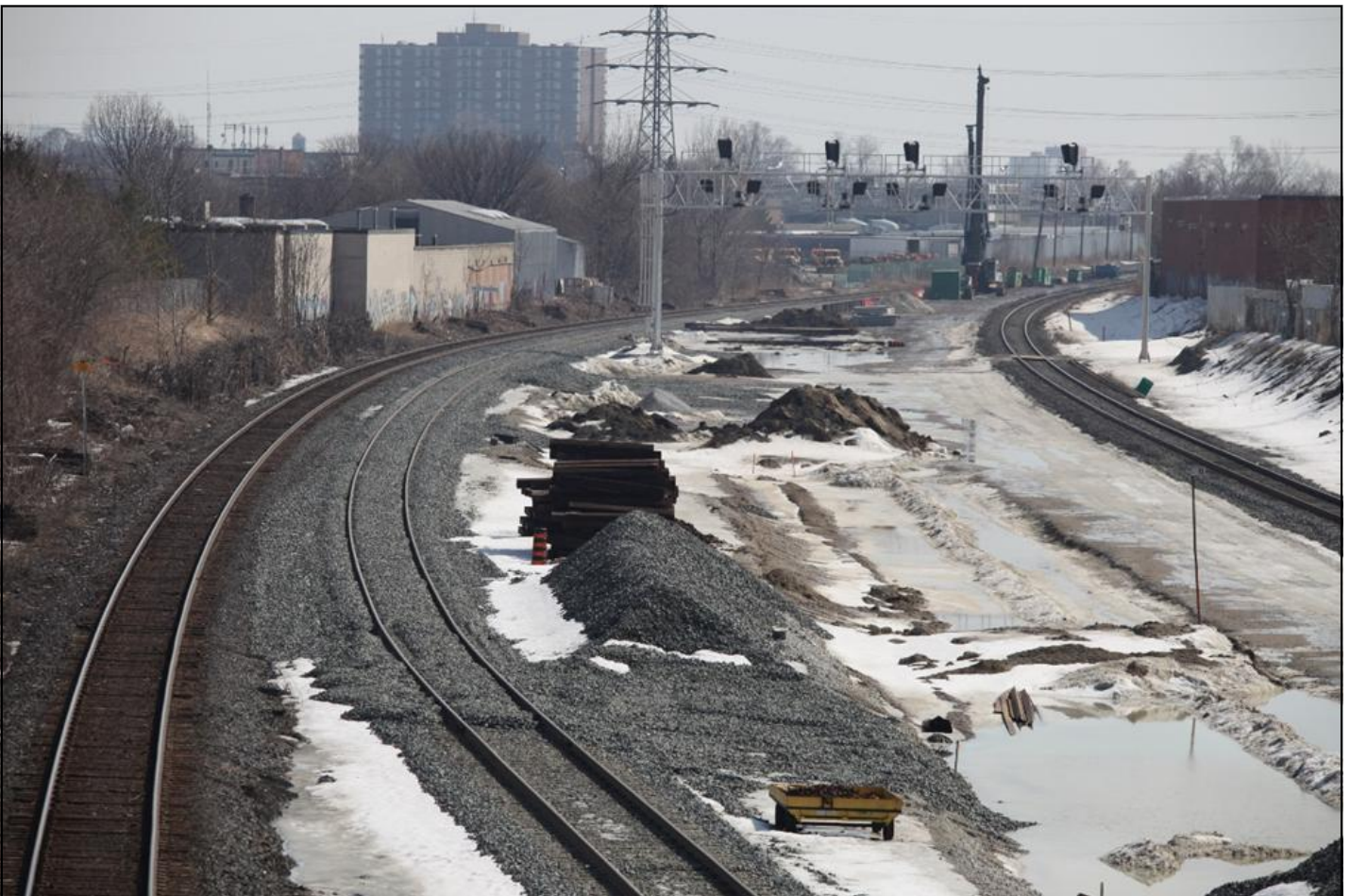
PHOTO 6 BELOW: New track being laid along the Union Pearson Airport line route. Eventually there will be four tracks in addition to the CP line on the right. Note: consistent colour of dolostone ballast under second track plus stockpiles.
